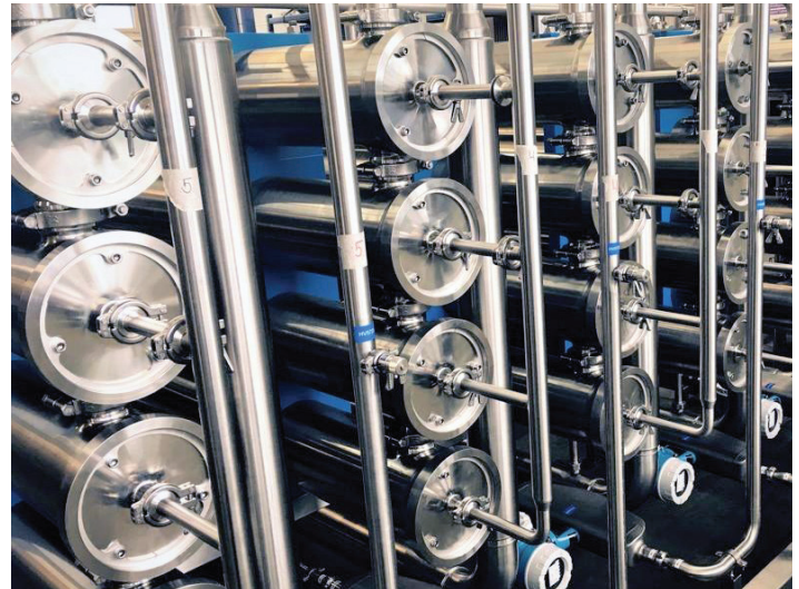
Figure 1: Heat sanitisable RO system. Image source MMS AG Urdorf Switzerland
