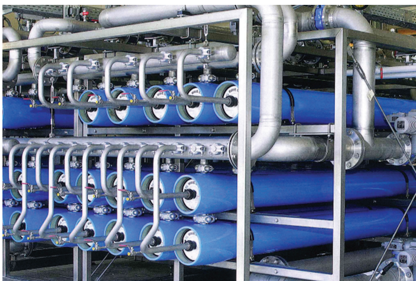
Figure 1: Low-pressure RO system at Löhnen drinking water plant
