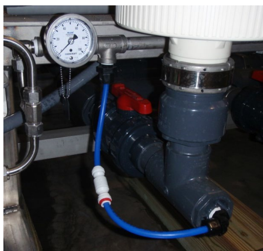
Poor location for air inject
