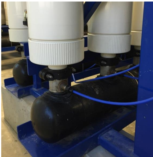
Good location for air inject
