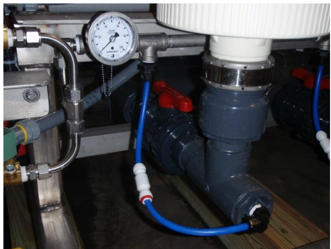
Poor location for air inject
