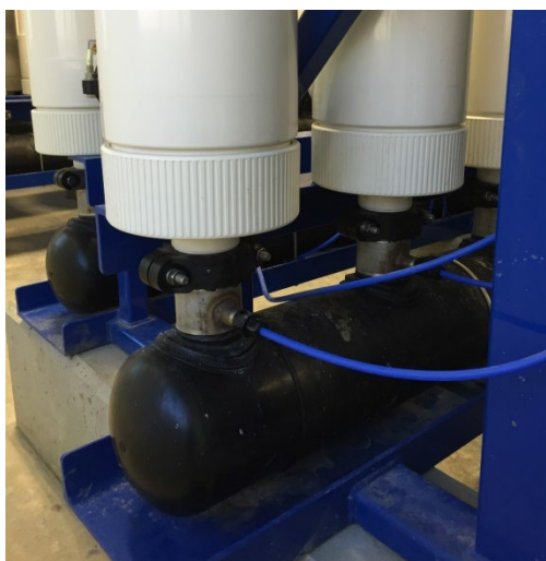
Good location for air inject
