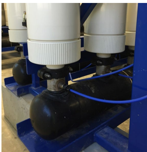
Good location for air inject
