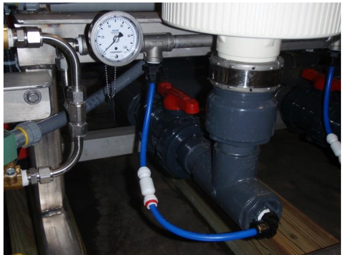
Poor location for air inject
