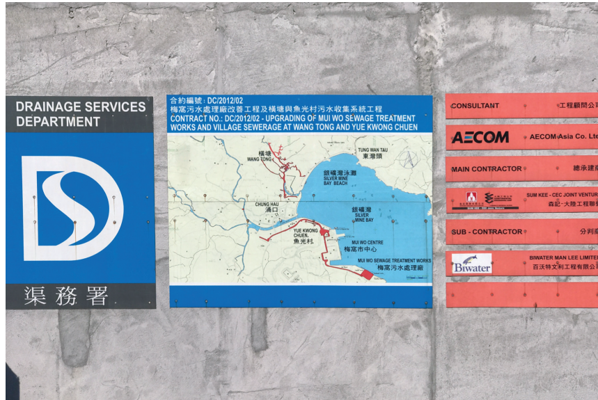
Figure 1: Mui Wo Sewage Treatment Facility
